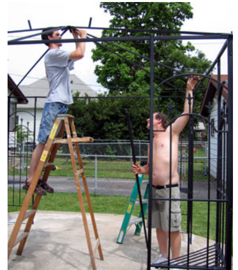
After all four corners were positioned, Chad & Dan begin installing the top frame that will hold the 'roof'
