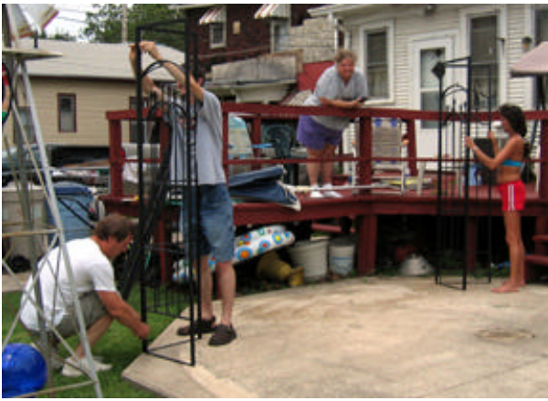
On July 3rd 2005, Dan, Tammy & Chad arrived with their sleeves rolled up ready to get to work installing our new Gazebo.
